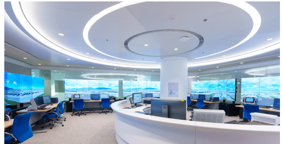
The upgraded system is capable of joint simulation training of the whole tower-approach-area control training process 已升級的系統能支援集合塔台管制、進近管制及區域管制整體流程的模擬培訓
